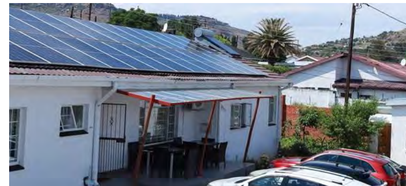
Foto: SolidarMed Lesotho - 30kW Solar PV System on health facility
